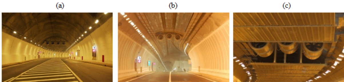
Figure 6: Details of horizontal signals (a), ventilation system at a junction (b), ventilation system with acoustic attenuators (c)
