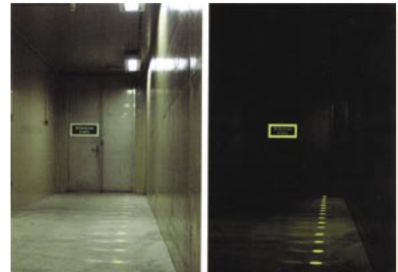
Figure 46: Example of cross connection with and without lighting. Note the photo-luminescent and self-adhesive dots on the pavement guiding to the door of the other tube.
