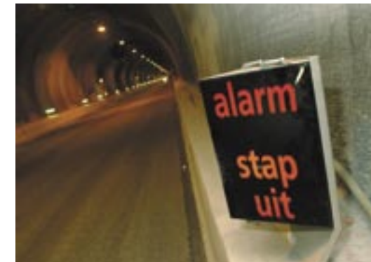
Figure 39: Pre-recorded dedicated alarm text message applied in the Westerschelde Tunnel (NL "stap uit" means "leave your vehicle" )
